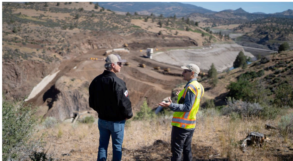
Governor Newsom at Klamath River dam removal project in Siskiyou County this week
